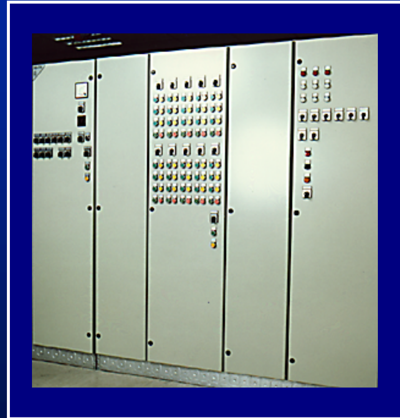
Operation- and Control Board
